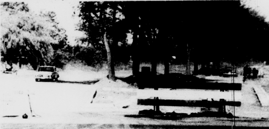
NEARING COMPLETION--With Shaw Lane widened to a tree-lined boulevard from Farm Lane to Harrison Road, campus residents and visitors will find rush hour traffic less of a nuisance and safer. The widening of the
