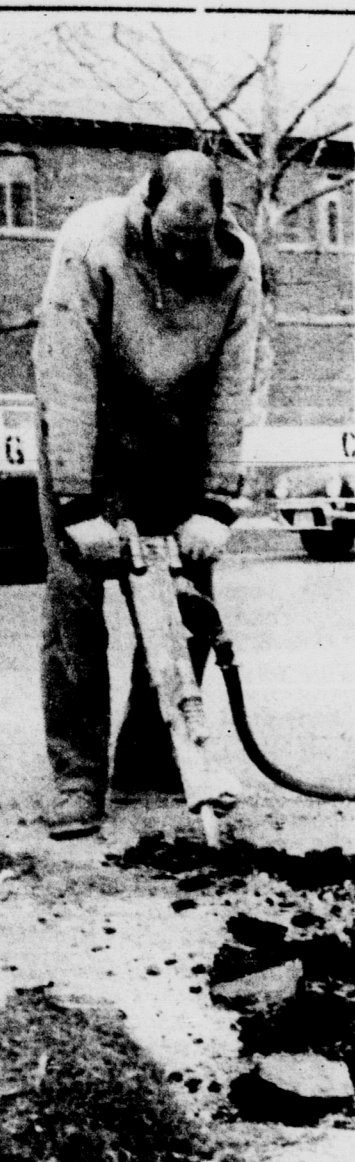
FIX-IT TIME—Steam leaks have resulted in disruption of sidewalk traffic near Berkeley Hall as maintenance crews have dug up the cement in order to repair the deeply buried pipes. State News Photo by Dave Joehrig.
