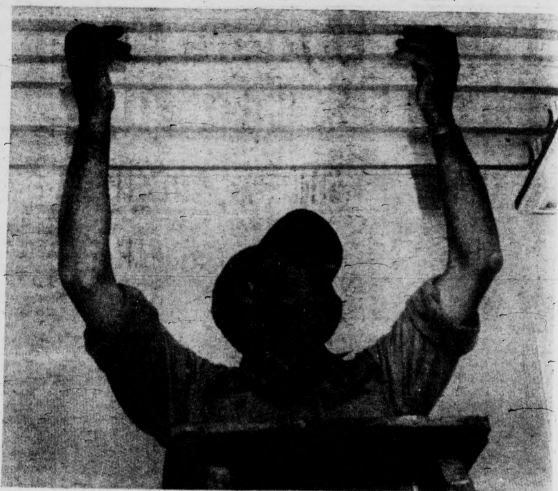
A WORKMAN places fluorescent lamps in fixtures just installed in Bessey Hall located across from the Auditorium.
