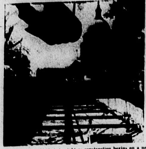
A CAPITOL ADDITION is in sight as construction begins on a new subway leading from the old and new Senate buildings to the Capitol in Washington. It will aid lawmaker's transportation.
