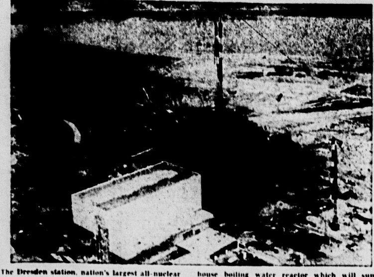
The Dresden station, nation's largest all-nuclear power plant, takes shape on the Illinois waterway southwest of Chicago. Steel sphere will house boiling water reactor which will supply power for the turbines housed in adjacent buildings.—AP Photo. (See related story, page 3.)
