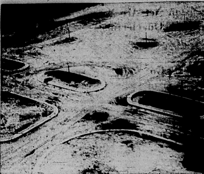
Above is the site of the new parking lot at Kellogg center. This unique lot will have shaded parking, and will accommodate several hundred cars. The landscaping and architect department, headed by Prof. Harold W. Lautner, is constructing the lot, which is due for completion in early September.
