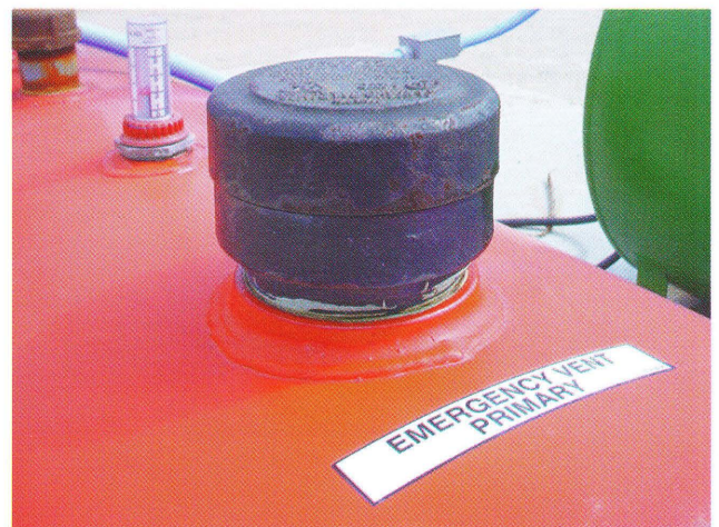
Fig. 5. Close-up of emergency vent.
