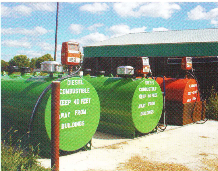
Fig. 6. Here are two double-walled tanks and one single-walled tank with secondary containment. The two emergency vents indicate that the two tanks on the left are double-walled tanks, while the single-walled tank has only one emergency vent (hidden).
