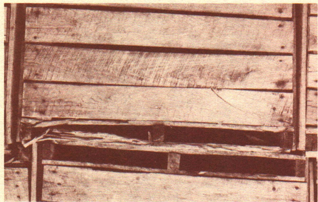
Damage caused by failure due to wood decay.
