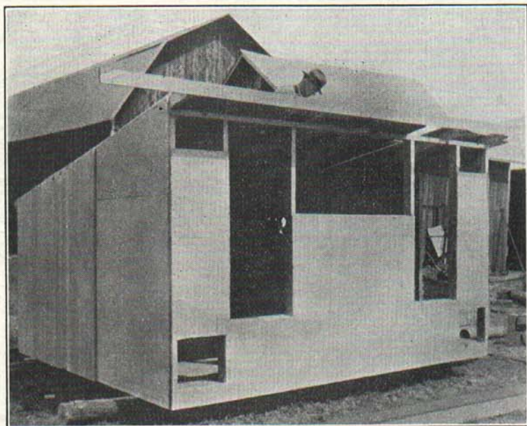
Fig. 2.—Shows method of applying insulation board with siding nailed in vertical position.
