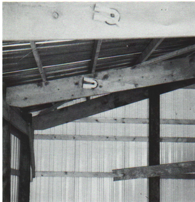
Figure 2 — One-2½ in. split ring was used on this joint where at least two rings should have been used.
