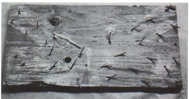
Figure 6 — A gusset plate from a building that failed. About a 10 to 20 percent glue contact area is apparent from the wood fiber failure. Glue did not squeeze out of this joint.
