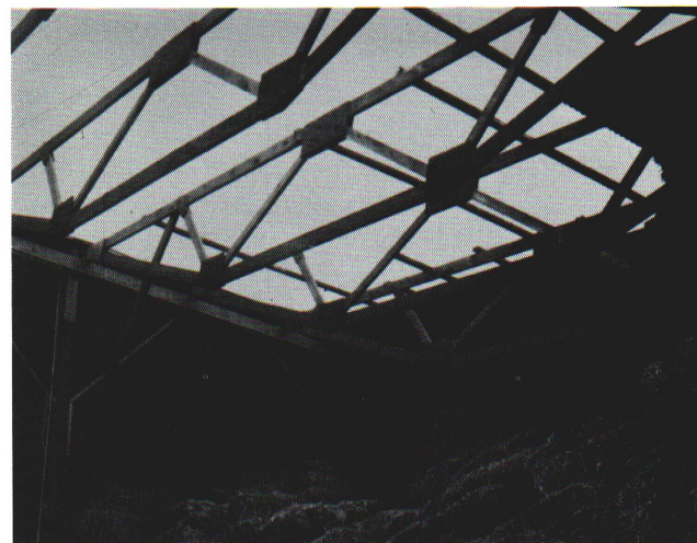
Figure 11 – Poor nailing of roof girts to trusses caused this section of roof to blow off during high wind.
