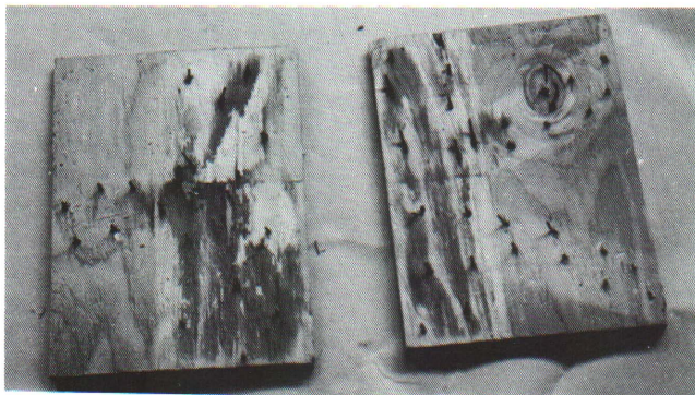
Figure 4 — Gusset plates taken from a truss showing the mold formed in the glue — indicates very little contact area.
