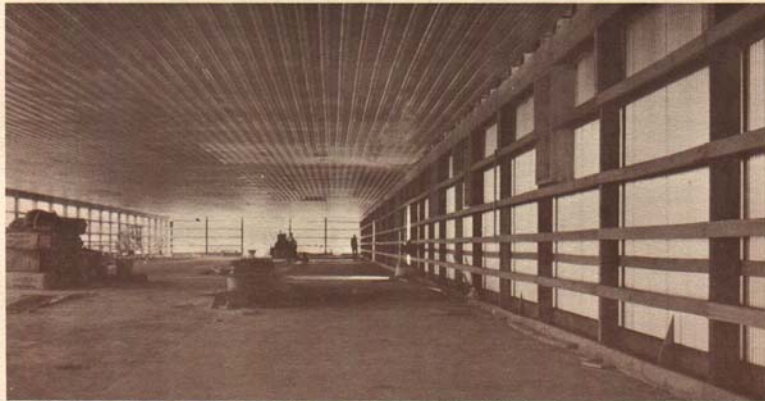
Fig. 17.—Square pole framing for a windowless poultry house. Building is lined inside and out with metal. Blanket insulation is placed in the wall horizontally.
