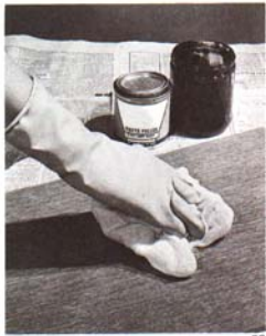
Finish wiping the filler, using cheese cloth with light strokes with the grain.
