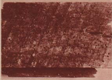
When adult Powder Post beetles emerge, some species leave small holes about the size of a pin in the surface of the wood; others make holes the size of pencil lead. Note the tunneling is to both wood and bark, but primary concern is the damage to the wood.
