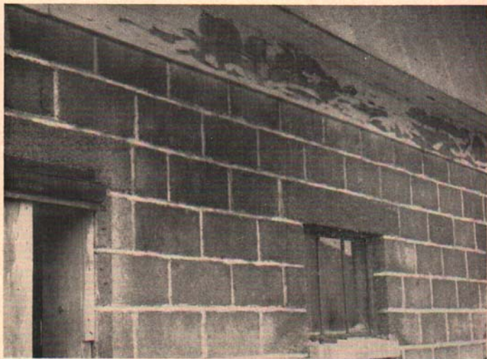
Fig. 1. The paint peeling under the eaves shows one of the effects of improper ventilation in this new masonry barn.
