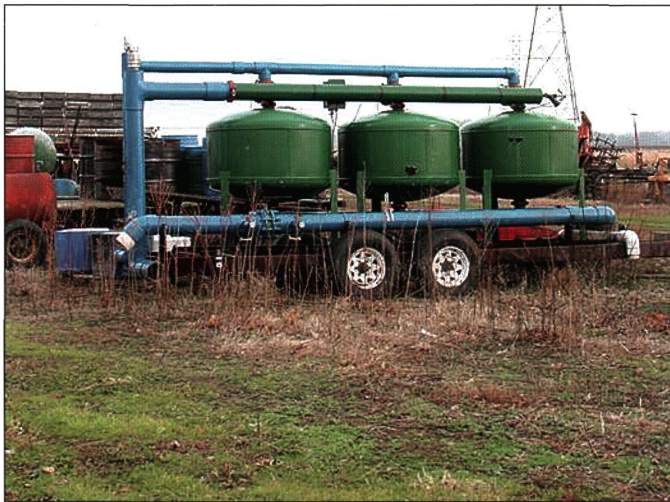
Fig. 11. Sand filter for irrigation water.
