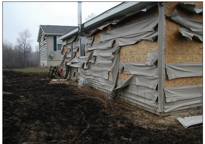
Figure 4. A wildfire in a grassy field melted the siding on this garage and home.
