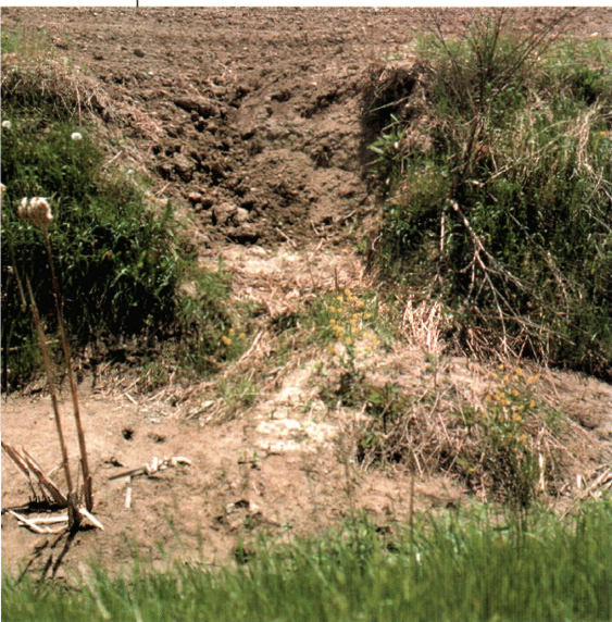
Ditch bank blow-out.
