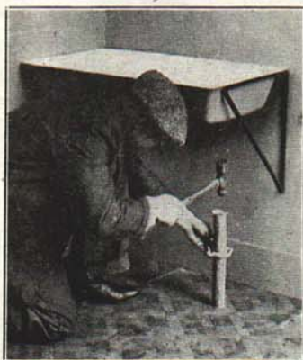
Figure 7: Lead pipe should be flanged to fit the pipe clamp.
