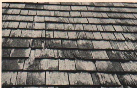
Fig. 16. Edge-grain shingles will not warp or curl even when badly weathered, thus reducing the fire hazard.
