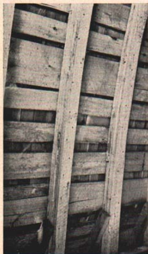
Fig. 14. A mediocre roof deck. The roof boards show numerous defects, and uniform nailing of shingles is difficult because of random widths and uneven spacing of roof boards.
