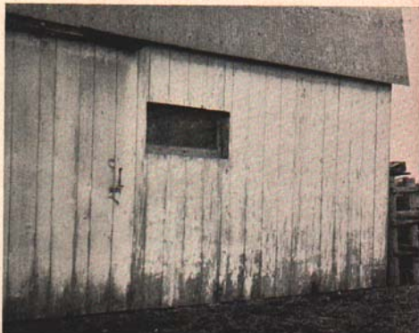
Fig. 9-d. The Jack pine siding already shows indication of decay at ground line after only one year of exposure.
