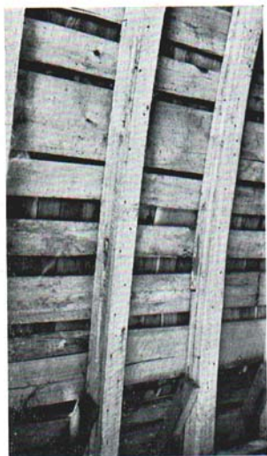
Fig. 14. A mediocre roof deck. The roof boards show numerous defects, and uniform nailing of shingles is difficult because of random widths and uneven spacing of roof boards.
