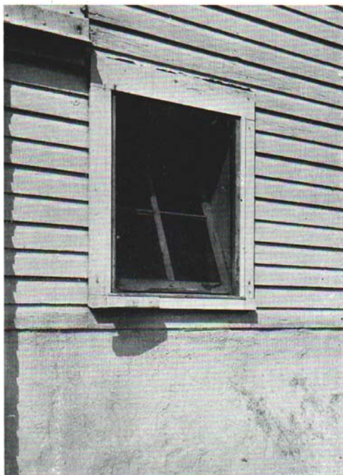
Fig. 8. Window construction without drip cap. This picture shows paint failure owing to moisture seepage around window frame and trim.
