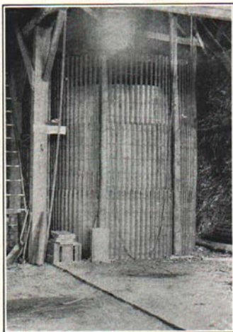
Fig. 3. A crib silo on a barn floor. Additional posts were placed under the floor to support the increased weight.
