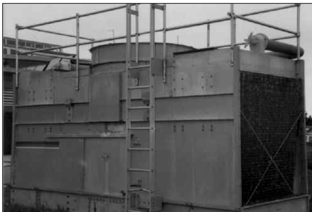
Induced draft-type cooling tower showing air intake vent and safety rails around the top of the tower.
