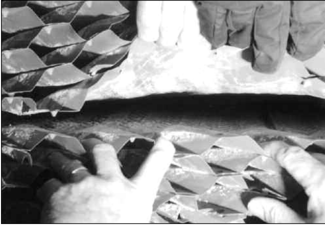
Close-up of cooling tower fill where microbial growths can accumulate and reduce system efficiency.
