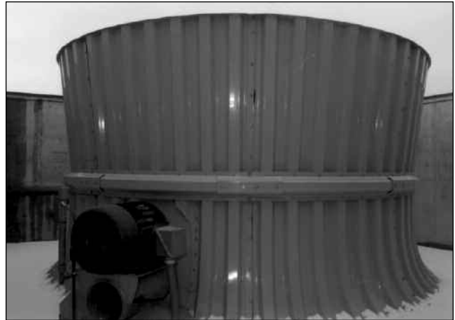
Exhaust tower on an induced draft cooling tower system.
