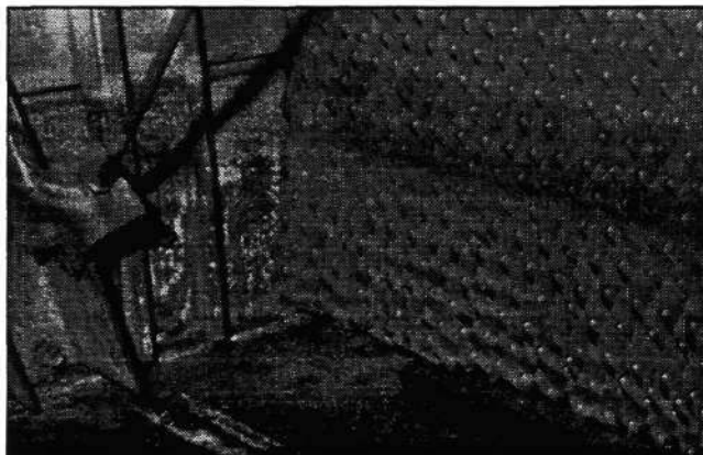
Two examples of cooling tower 'fill' through which water circulates.
