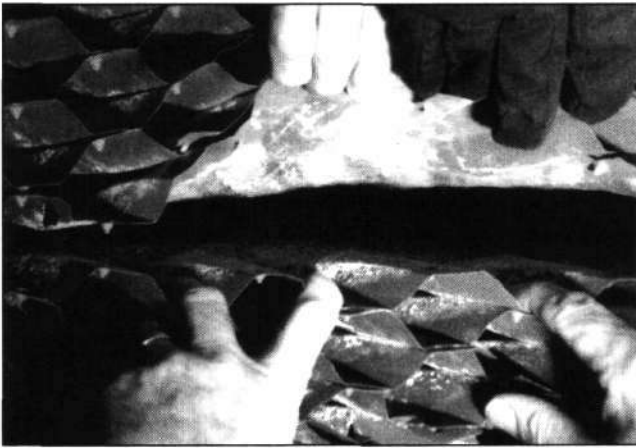
Close-up of cooling tower fill where microbial growths can accumulate and reduce system efficiency.
