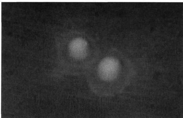
Improper application of biocide tablets. Tablets of formulated biocides should be metered and fed, or suspended in the systems water flow rather than dropped in the basin as shown here. Note the dark pock marks in the concrete surface damaged by previous applications.
