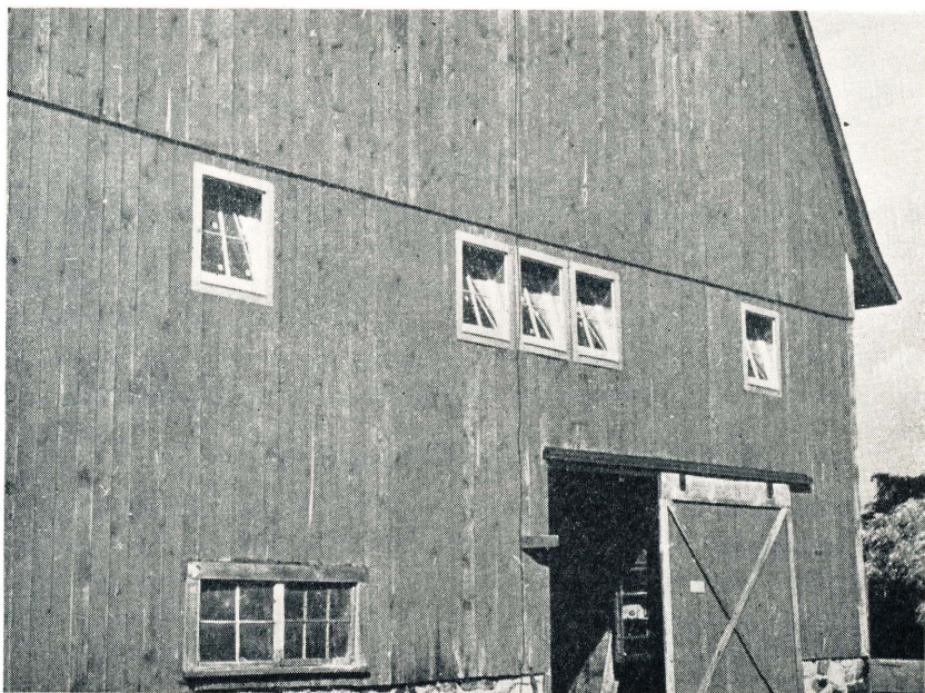
Fig. 17. Changing the hay mow over into a laying house. Note the use of galvanized window sash, which eliminates much labor in the framing of the window.
