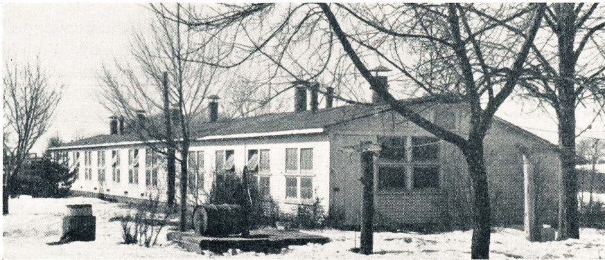
Fig. 16. A 20' x 80' laying house that has given satisfactory results for the last 18 years. The entire roof, despite careful attention, must be replaced at once.
