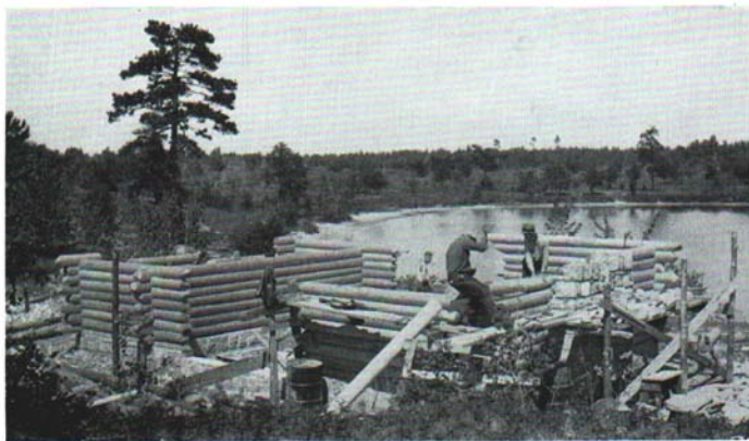
Fig. 1. A well chosen cabin site commanding an excellent view. Peeled jack pine logs are being used. (Photograph by the U. S. Forest Service.)
