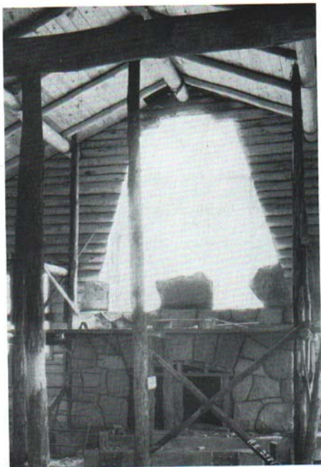
Fig. 19. Partially completed fireplace showing the placement of corner stones, framing for the fire-box arch and scaffolding.
