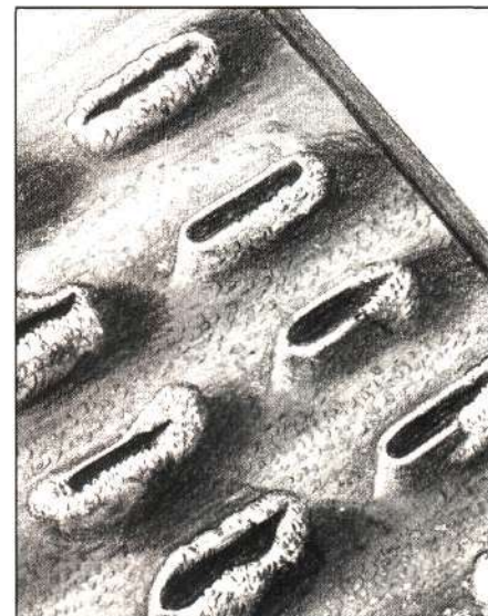
Severe radiator corrosion
