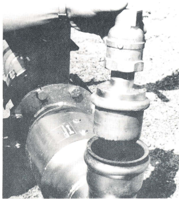
Removable vacuum relief valve serves as a port to inspection check valve.
