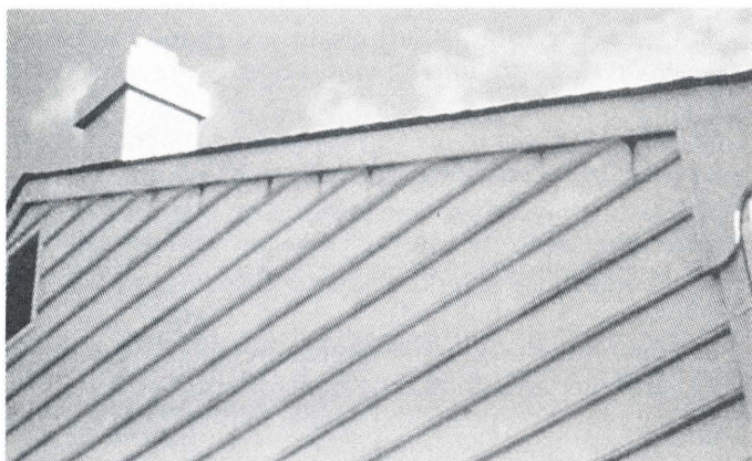
Figure 6.20. Carpenter bee damage.
