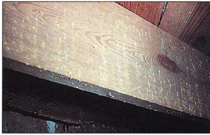
Anobiid beetle damage
