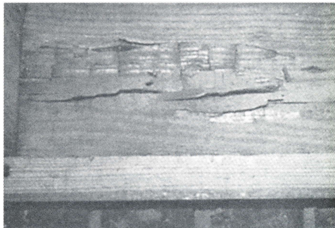
Figure 7.2. Wood damaged by Poria , with apparently sound surface and severe rot below surface.
