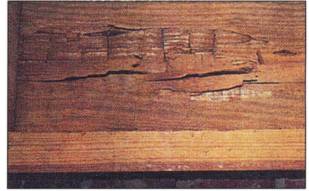
Wood damaged by Poria
