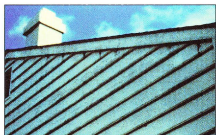
Carpenter bee damage
