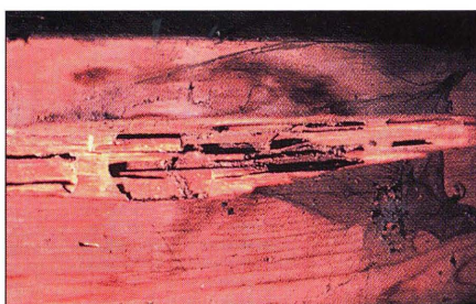
Subterranean termite damage to wood
