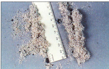
Carpenter ant shavings
