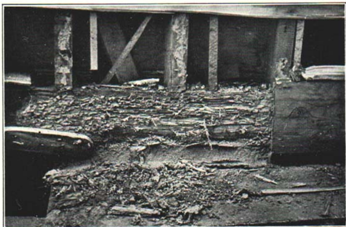
Fig. 5. Foundation destroyed by termites.
