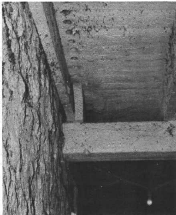
Figure 12. Two-inch diameter holes drilled in a ceiling to approximate a slot inlet.
