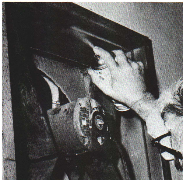
Figure 3. Repainting a fan housing after it has been cleaned and the bare spots have been primed. Keep a record card on fan maintenance near the fan.
