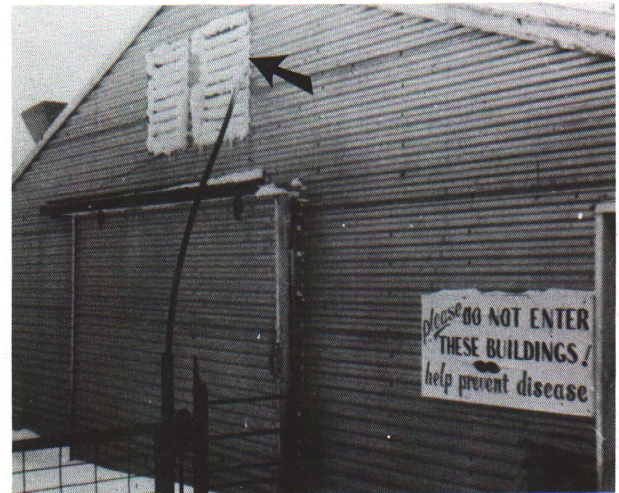
Figure 10. The variable-speed exhaust fan operated at too slow a speed in this farrowing barn. High winds sucked moist air from inside the barn back up through the ceiling inlet into the attic space. There it condensed into frost.
