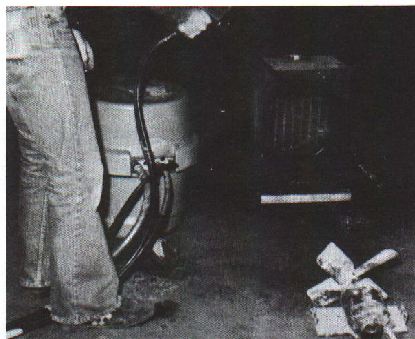
Figure 8. A pressure-washer being used to clean out the fins of an air heater. Note the fan is removed, as it has an open motor.
