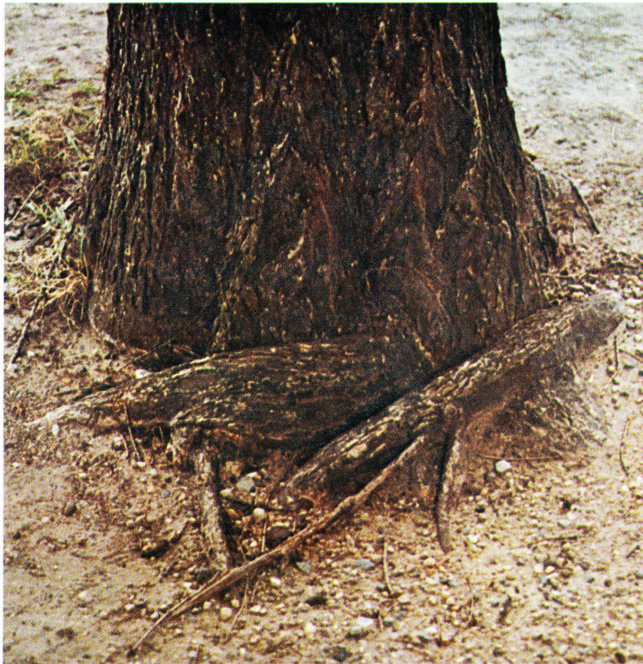
Fig. 2. Aboveground girdling roots. Two roots that are pictured encircle the base of the tree which may clog or stop nutrient and water flow in the tree. Often girdling roots are below ground and not visible unless exposed by digging.
