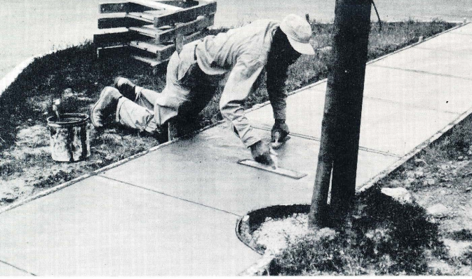
Fig. 7. Sidewalk with arc or curve to save the tree.
