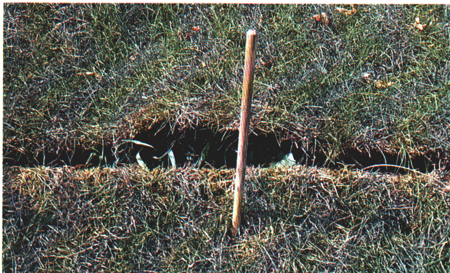
Sod can be staked to prevent slippage off of a slope., In this case the sod was stretched during installation and gaps were formed once the sod dried.
