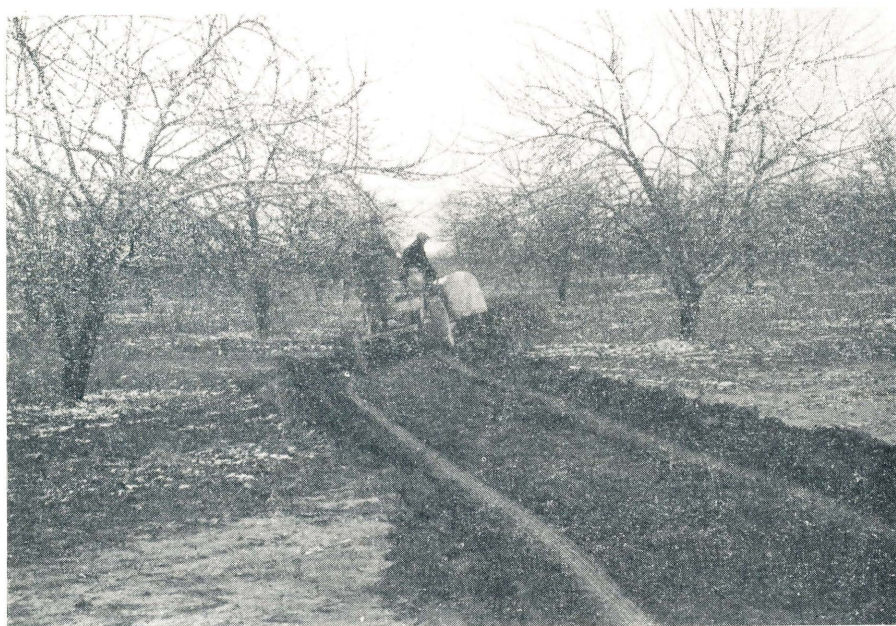
Fig. 5. Showing the construction of a diversion terrace in an established orchard. In some cases it is necessary to remove an occasional tree in order to properly construct such a terrace.
