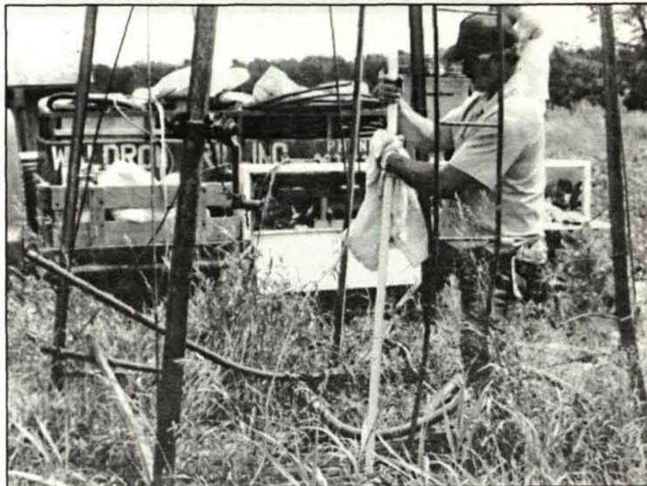
Dan Waldron, owner of Waldron Drilling is shown pumping bentonite slurry into the well casing of an abandoned well located in a soybean field on the Hugh Roberts farm near Carson City. Once the casing was sealed with the bentonite, the well casing was cut off three feet below the surface. The windmill and rigging are to be removed and the well pit filled with soil so the land over the old well can be farmed without causing the groundwater to be contaminated.
