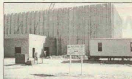
The new processing plant, still under construction, will eventually be able to process 200 tons of specialty crops per day.
