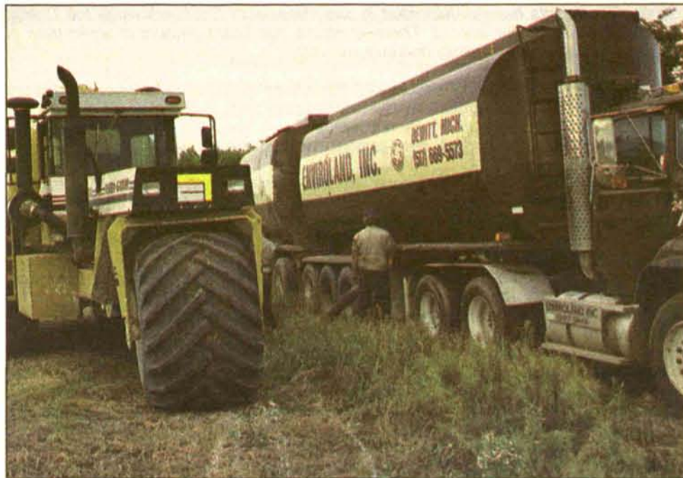
Enviroland workers load a spreader with liquid lime from one of their transports.
