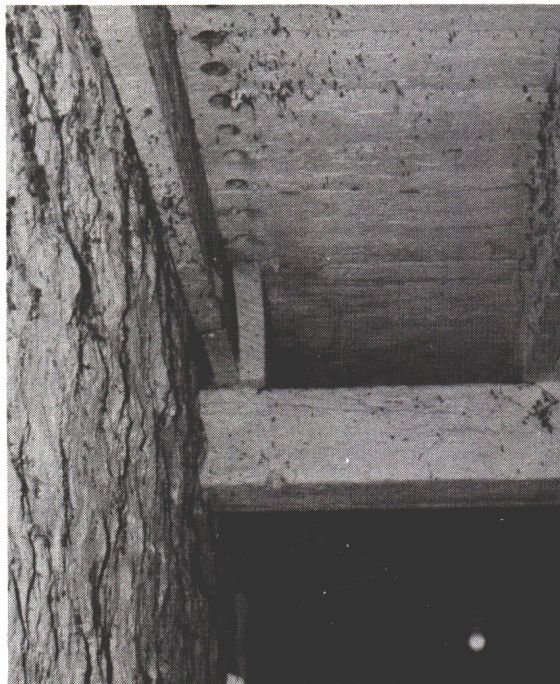
Figure 12. Two-inch diameter holes drilled in a ceiling to approximate a slot inlet.
