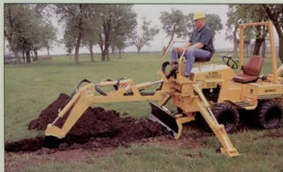
Vermeer increased the productivity and versatility of its V-3550 riding trencher with the addition of a backhoe.
