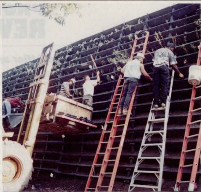
Each of 5,300 built-in flower boxes is hand planted: shade-loving plants on the north, an assortment of shrubs and flowering plants facing the freeway.
