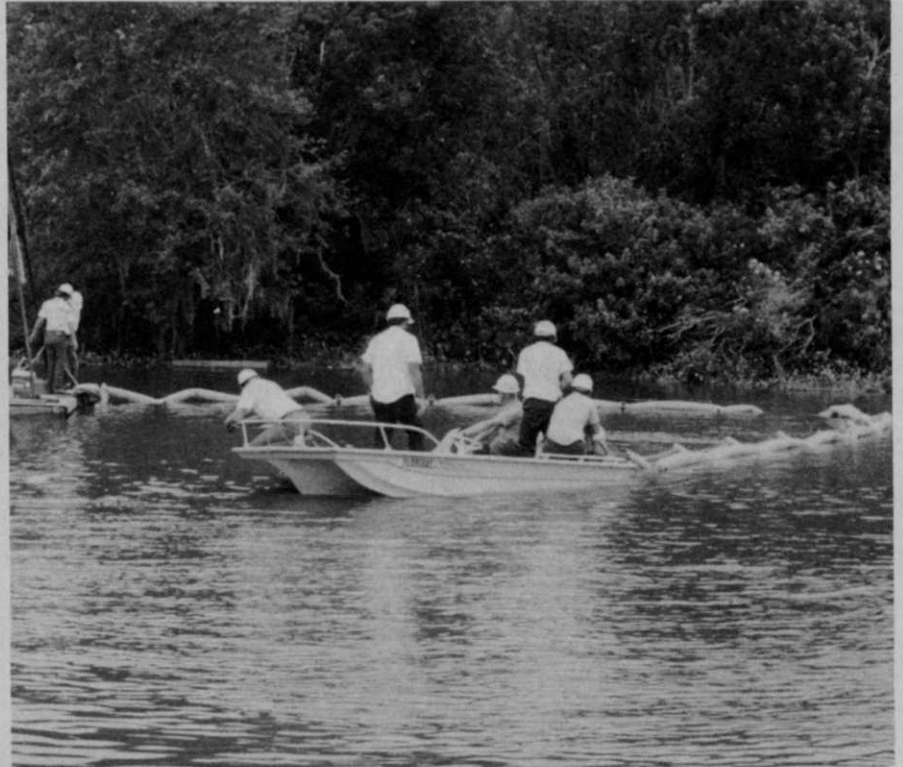
Work crews install a barrier by floating it into place and then tying it down to concrete blocks. Barrier is easy to maneuver.
