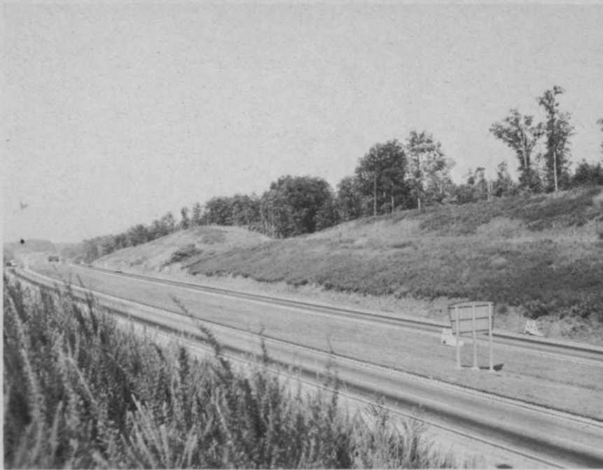
Weeping lovegrass and sericea lespedeza control erosion. Woody Plants become established on slopes.
