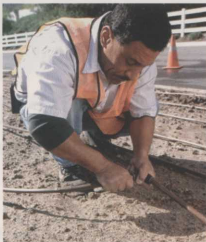
Once the lines are completed, the installer can flush them out and check the emitters.
