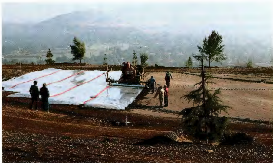
Putting green soil sterilization is important just prior to establishing the turf cover.
