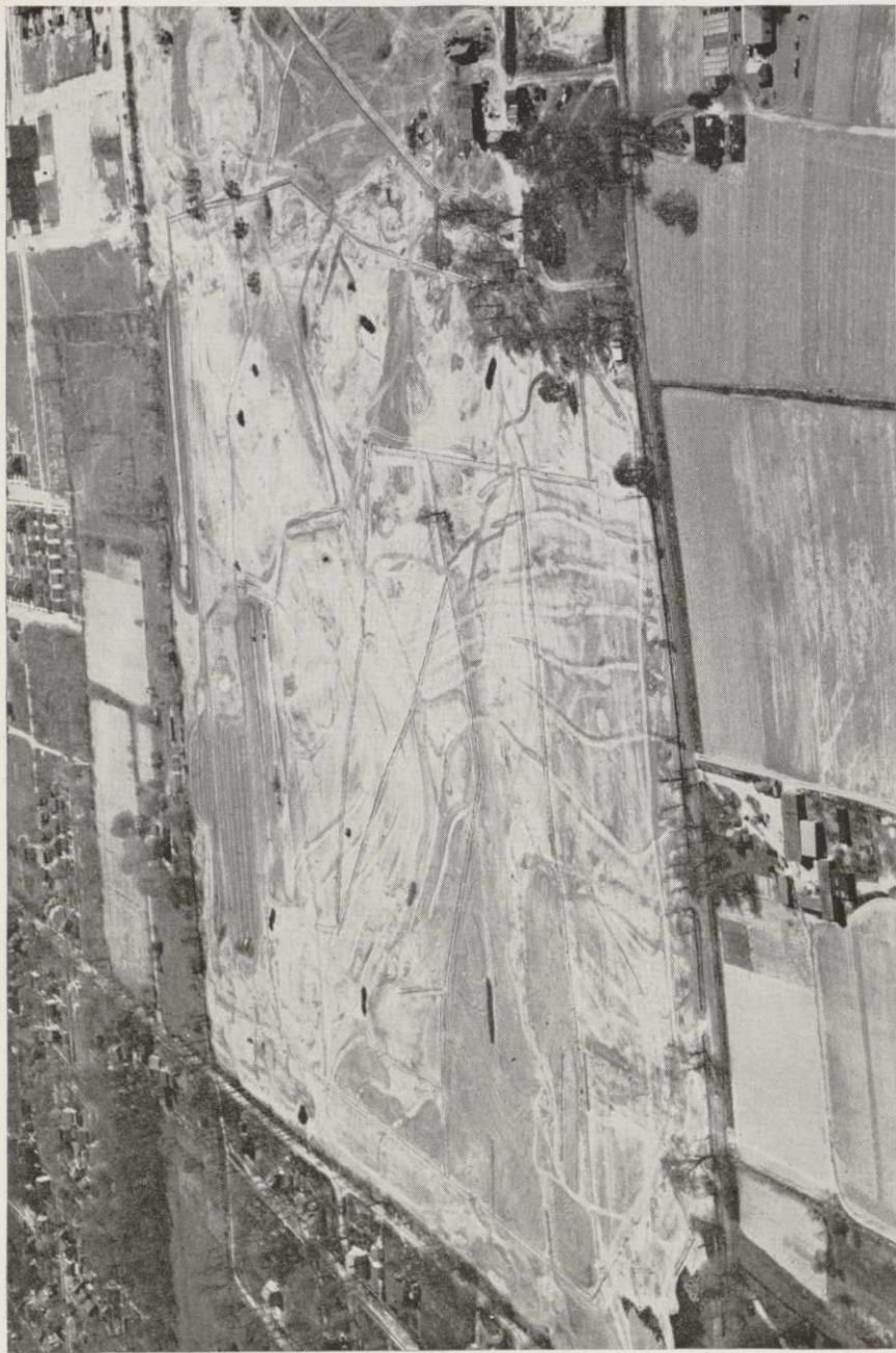
BAYSIDE COUNTRY CLUB, Bayside, Long Island, N. Y.—a truck garden being transformed into a marvelous golf course for the Meyer-Cord Realty Corp. Laid out by Dr. Alister Mackenzie, architect; built by the Wendell P. Miller Organization. A complete fairway irrigation system and five tons of Scott's Seed insure good turf.
