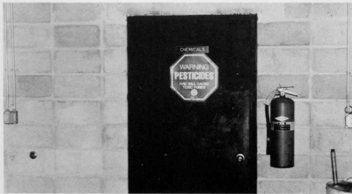
Highridge C.C. exemplifies properly locked metal chemical room door with signs posted and fire extinguisher.
