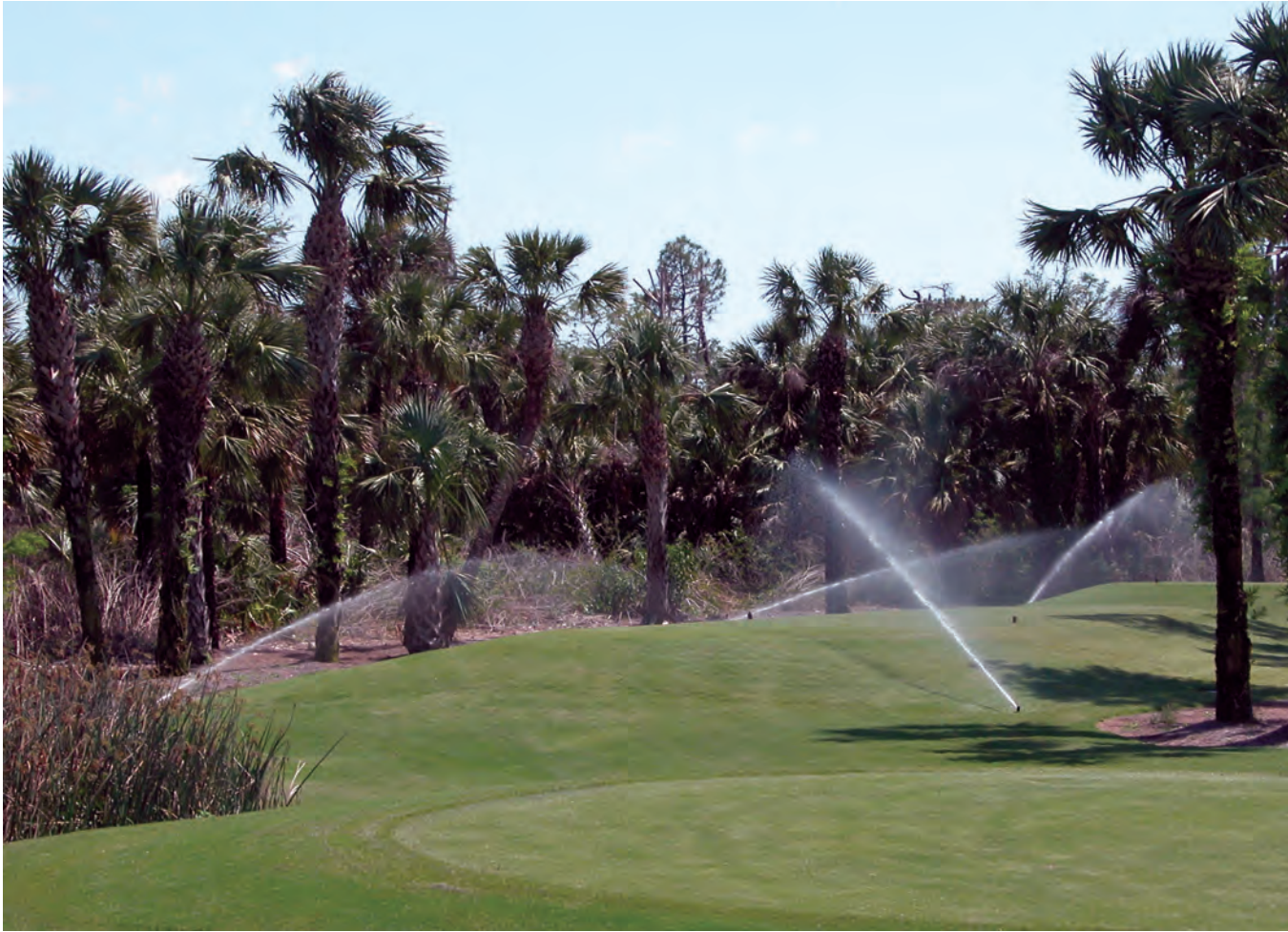
Regularly check irrigation head nozzles and operation for efficiency and conservation. Photo by Joel Jackson.
